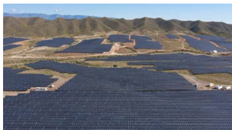
Photovoltaic park LaCabrita - Almería, Spanien 122,000 PV modules, in operation since 2021
