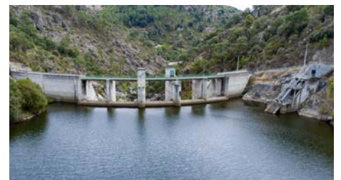
Hydropower Sagres, Portugal 21 plants, commissioned 1951-2006
